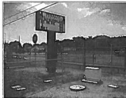
The circular grinder pump lid for Peralta Elementary is shown in the above picture. The grinder pump underneath the ground is part of the Bosque Farms low-pressure system that was designed by Molzen Corbin.
