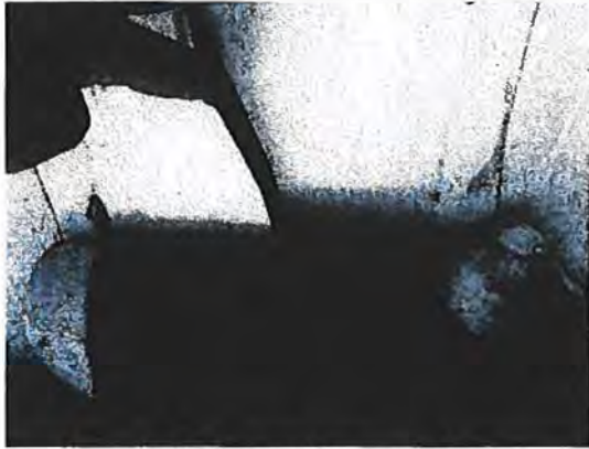
Failing, previous repair.
