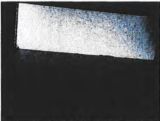
Leaks at skylights
