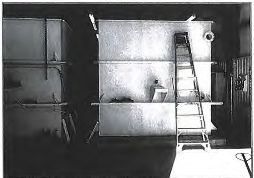
Molzen Corbin helped the Village of Chama to improve system redundancy and increase capacity of their surface water treatment plant by installing a second treatment train.
