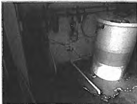
Molzen Corbin's experience with the Taylor Well Field and history of water treatment work can be beneficial in addressing improvements to onsite disinfection systems.
