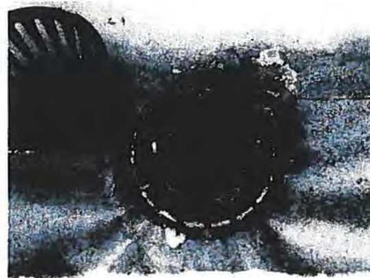
One of the leaking drains.
