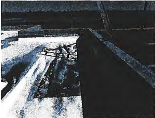
Worn TPO, low spots, leaking drain, and failing
