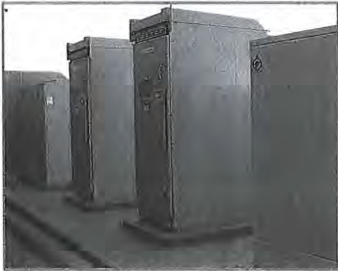
Molzen Corbin provided complete electrical design for new Booster Stations # 4A and #5A at the new Buckman Water Treatment Plant. The booster stations are housed in a single structure and consist of a combined 800HP of booster pumps powered by a 3,200A switchboard and feed from a redundant set of 2MVA service transformers.
