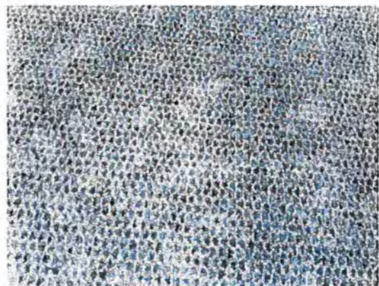
Worn TPO on a dry portion of roof.
