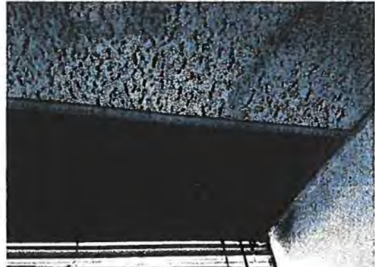
More damage from leaks.
