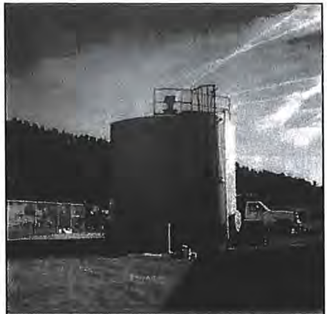
Molzen Corbin assisted the City in increasing capacity at Well No. 2 in the Taylor Well Field, including installation of new water transmission pipeline.
