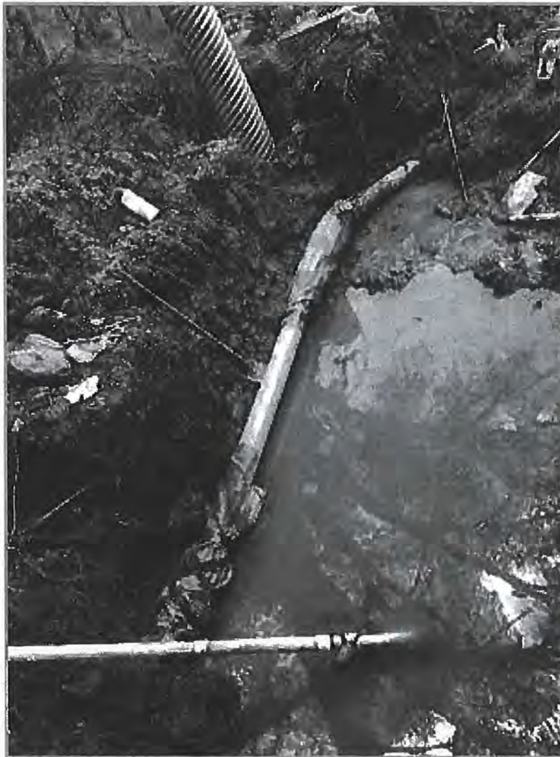
Molzen Corbin recently completed the Taos Street Waterline Repair under the Gallinas River.
