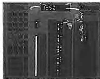
Molzen Corbin has provided recommended improvements to the control system to allow for automated control.
