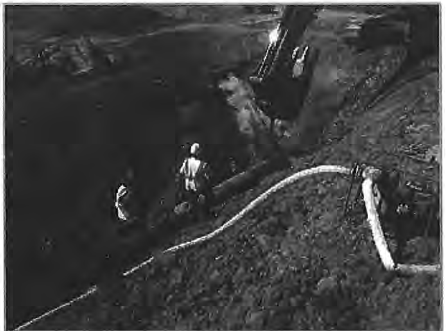
Molzen Corbin recently completed the Medite Waterline Repair replacing large diameter concrete cylinder pipe with ductile iron pipe.
