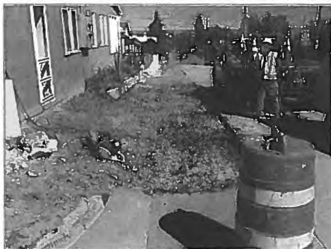
Molzen Corbin assisted the City with the design and construction of the New Mexico Avenue Effluent Line.
