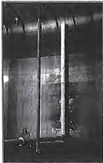
New Interior Piping at the Cabin Site Tank (2017)
