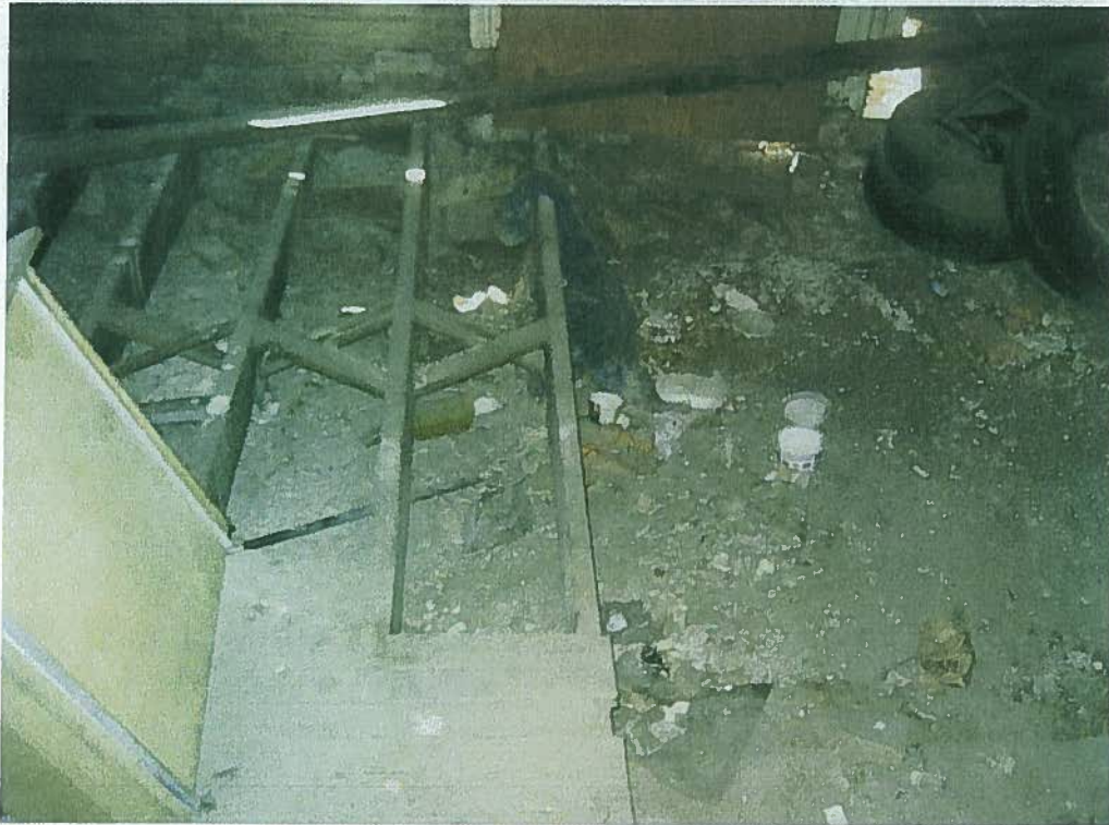
Photo 4. Location of filled in basement
