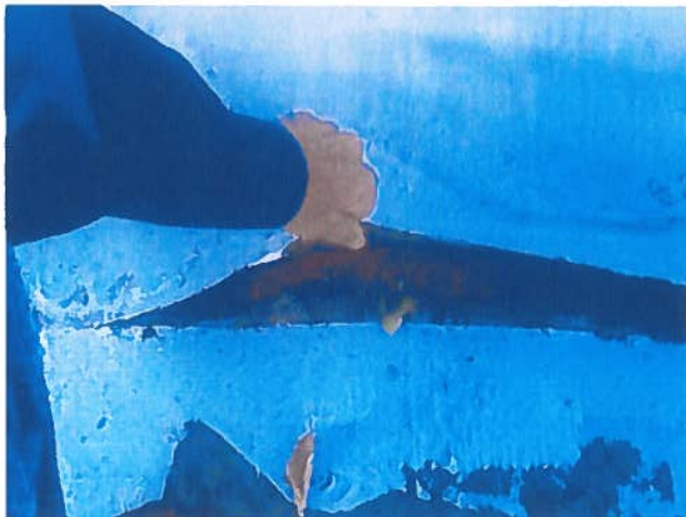
There are multiple sections that the seams are not glued or welded, but totally wide open to water and weather.
