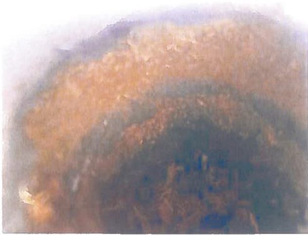
All layers will be torn off to the deck. ISO insulation will be replaced and a slope system For proper water runoff
