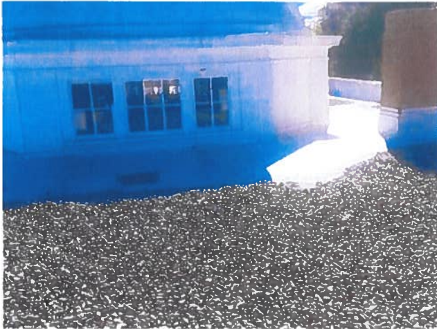
The roof system currently on this building is a 4 layer of insulation PVC liner. with River Rock to keep the liner in place.
